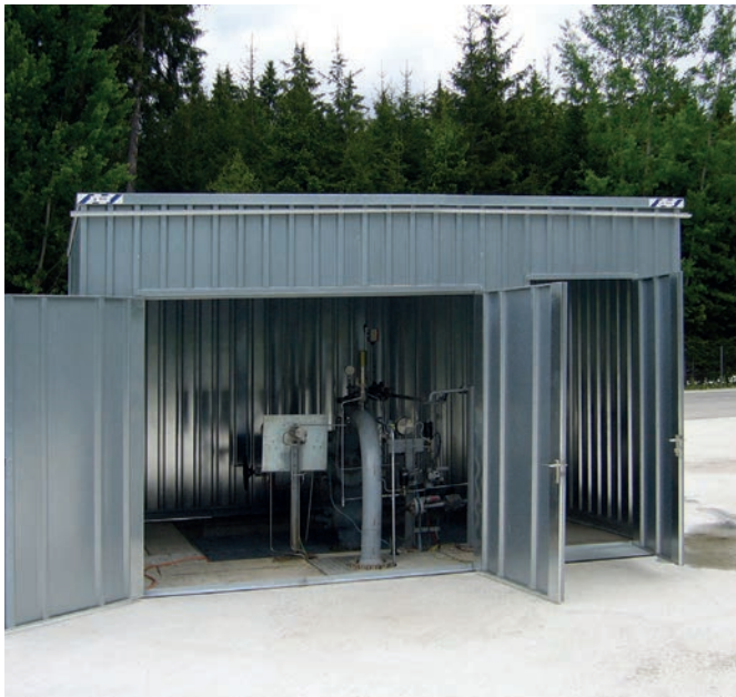
Gas pump housing
